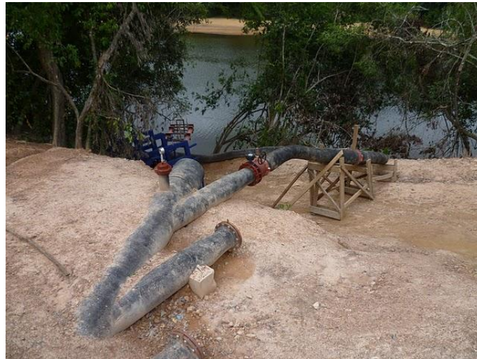
Addax pumping station on the River Rokel. © BFA
